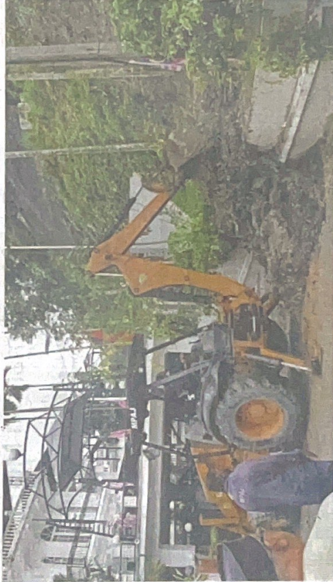
An excavator deployed by MPAJ to clear soil from Persiaran Desa Ampang 4.
